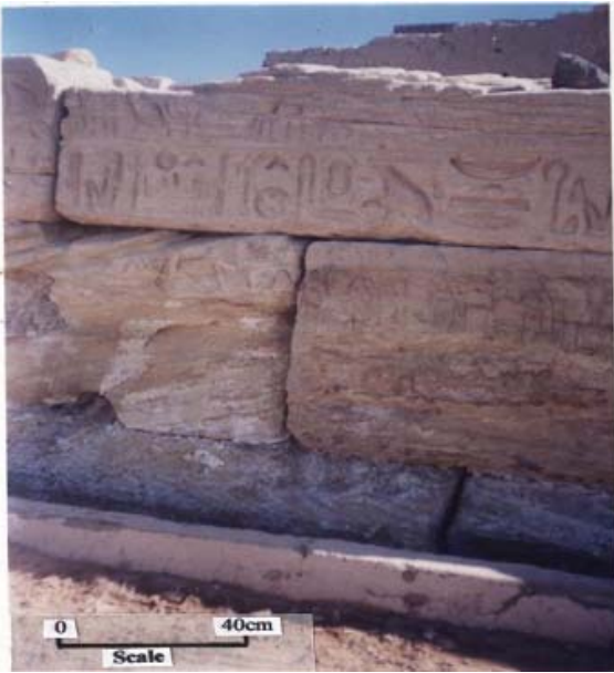
Figure 4: Severely weathered sandstone basal courses at West facing wall side of the first pylon (parts of investigation numbers 1 and 2), Seti I Temple.
