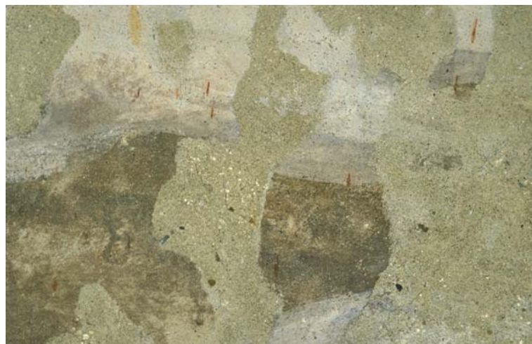
Figure 4: Facade paintings of Parz, detail with complete loss of the painted surface corroded into the plaster-layer
