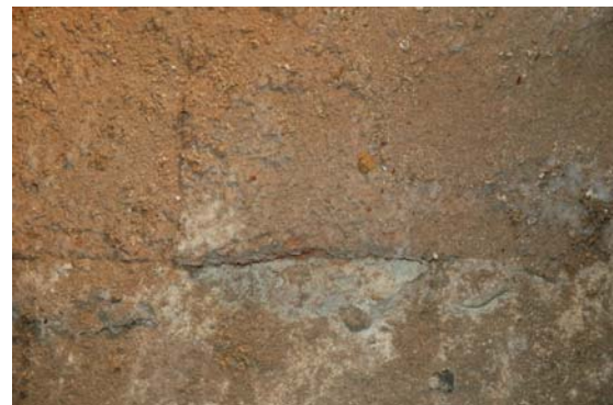
Figure 7. Visible efflorescence at the upper side of the vault.
