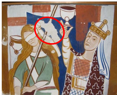
Figure 2. The wall section. Severe salt damage inside the red ring.
