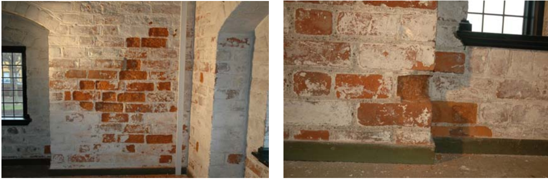
Figure 4. Deteriorated corner above the birds room. (a) Direction south-west (b) Direction north-west.
