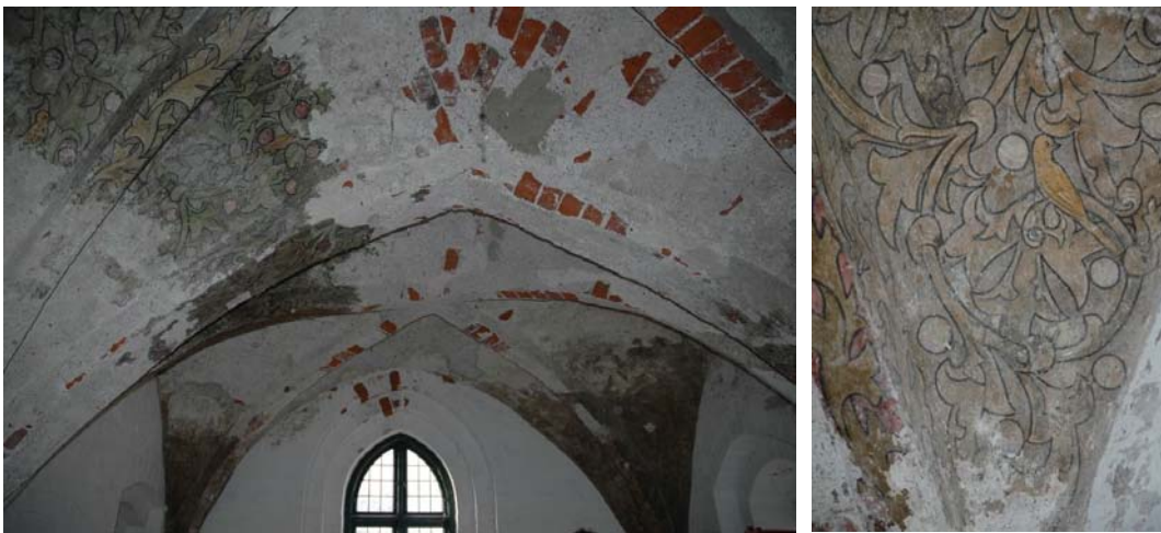
Figure 1. Extensive deterioration of the painted vault in the so-called Birds room in Vor Frue Monastery, Helsingør, Denmark. (Left) an overview (Right) a detail.
