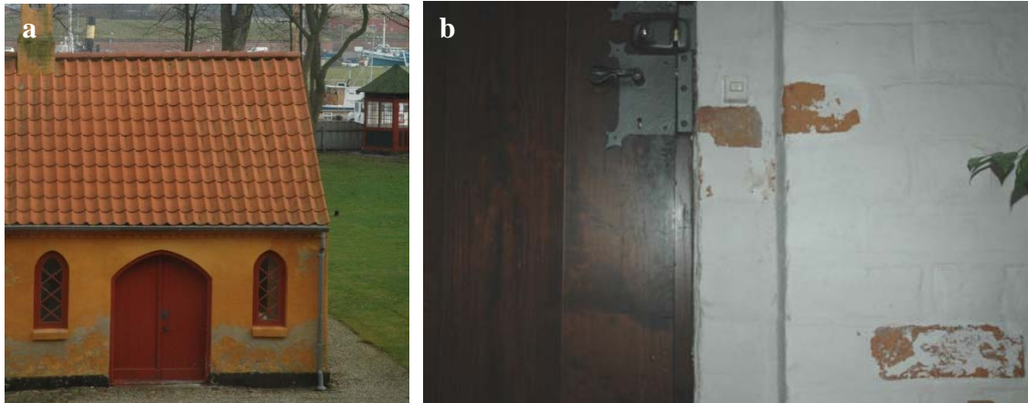
Figure 2. Plaster peeling (a) Traditional salt induced plaster peeling in a belt at approximately the same distance from the ground (b) Peeling of the lime wash in front of some specific bricks. In both cases the result is increased maintenance.
