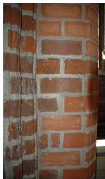
Figure 1. Picture of the pillar to the right of the altar in Sct. Mariæ Church, Helsingør, Denmark. Replacement with Falkenløwe bricks of deteriorated bricks have been carried out. Color variation is visible.
