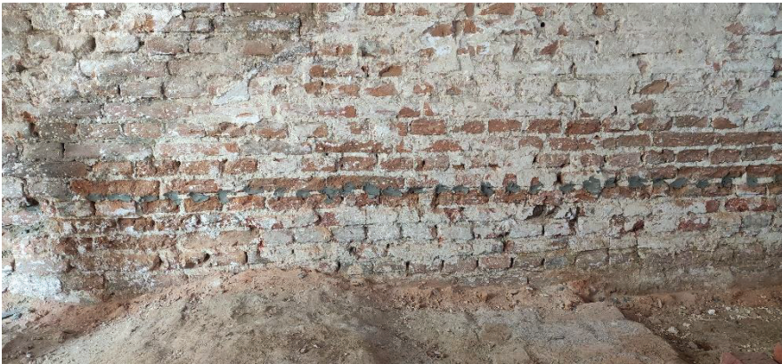
Figure 2: The stable wall showing the drill holes used for the injection with the damp-proofing agent after they were plugged with hydrophobic cement.
