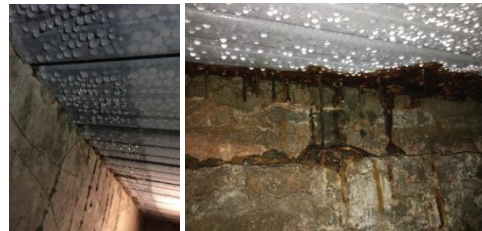
Figure 4: Left image shows condensation on the Bondek at the historic masonry wall side. The condensate water could lead to more water being absorbed by the historic wall. Right image shows the corrosion of the galvanised steel of the bondek especially where the deck butts the wall.
