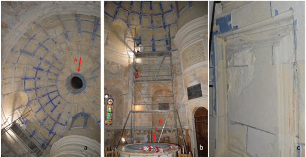
Figure 1: Interior of the chapel (a) view of the overhead dome, the arrow (A) indicates the oculus at the peak. (b): southern part of the chapel, the arrow (B) indicates the oculus on the floor of the chapel. (c): details of natural stone decay, granular disintegration, powdering and scaling are seen in the chapel. (Picture ECMH)
