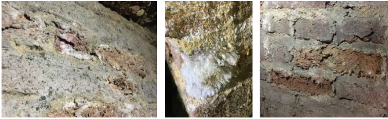
Figure 3: Left image - Efflorescence on the surface of the bricks accompanied by flaking or stratification of the surface layers. Middle image - Large crusts of salt crystals which have crystallized out from the surface of the bricks. Right image - Typical symptoms of friable clay and flaking of the bricks caused by salt crystallization.
