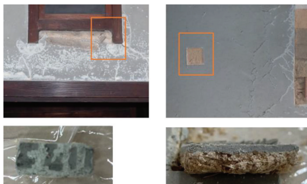
Figure 7 Sample and the collected part (upper-left: the collected part of sample A; bottom left: sample A; upper-right: the collected part of sample B; and bottom right: sample B where the deterioration is not evident)
