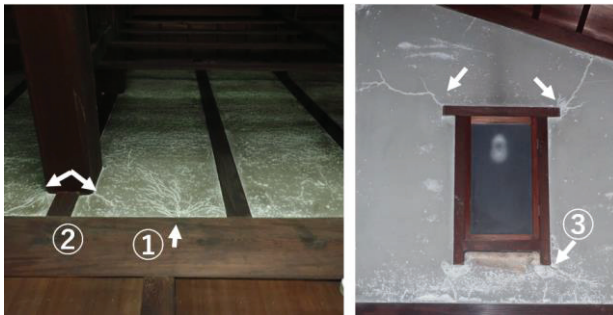
Figure 5 Linear deterioration (left Figure 2i, right Figure 2d)
