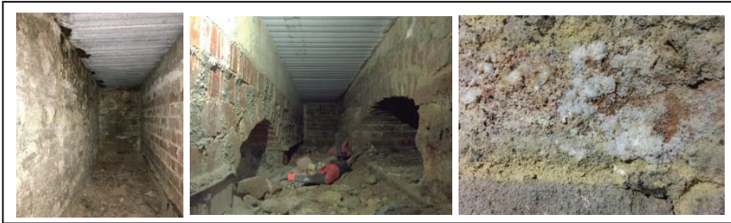
Figure 2: Typical view of a narrow space between the old and new masonry walls. Note also the corroded Bondek slab along the side with the historic masonry wall.
