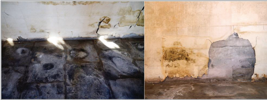
Figure 1: Indoor damages of building material: salt damage of floor bricks, cracking and mildew of wallpaper.
