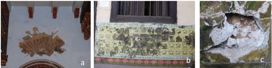
Figure 2: a- example of redistributed salt damage on a mural above an internal window; b- concentrated salt crystallization damage on dado tile below an internal window; c- close up view of damaged glazed tile
