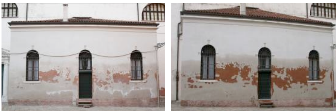
Figure 1: A building in Venice, two years apart. Does the reality of the degradation patterns fit to the theory of salt transport and crystallisation
