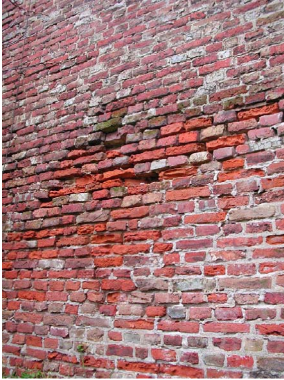
Figure 2: Damage occurring on the west wall of the tower
