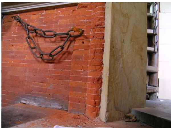
Figure 3: Powdering of the brick in one of the master proofs on the 1 st floor of the tower
